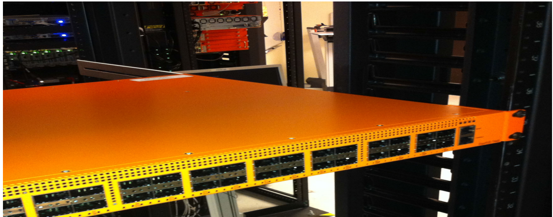
Figure 3-3: Front View of the Mounted Node to the Four-Post Rack
